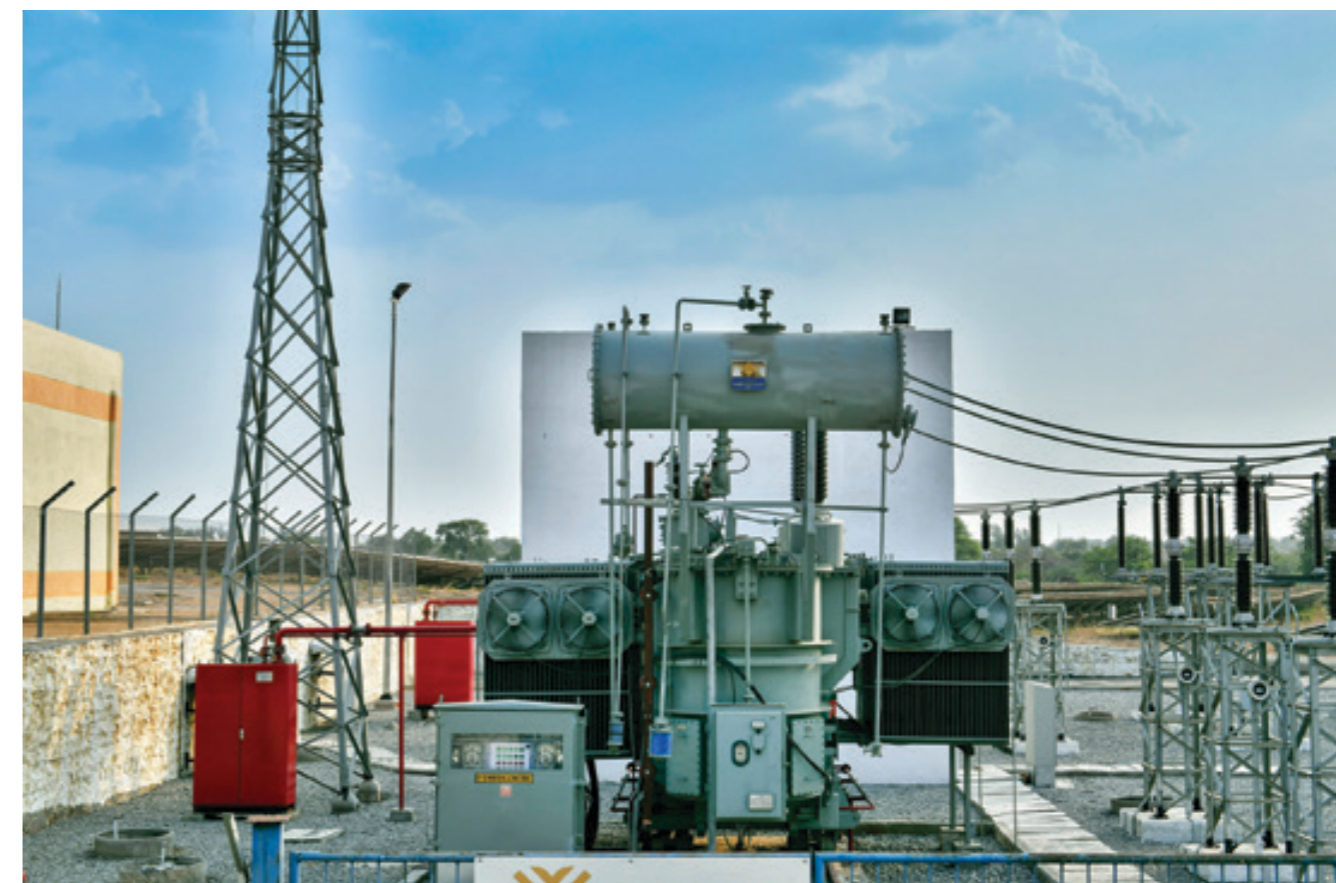
A substation in Telangana
