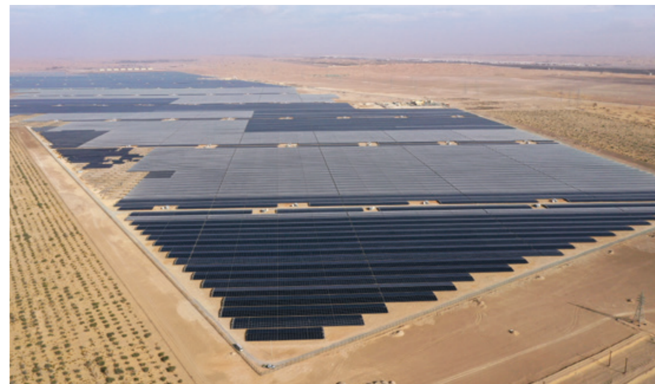
1,177 MWp Noor Abu Dhabi Solar Power Plant, the largest plant built by Sterling and Wilson Renewable Energy Limited
