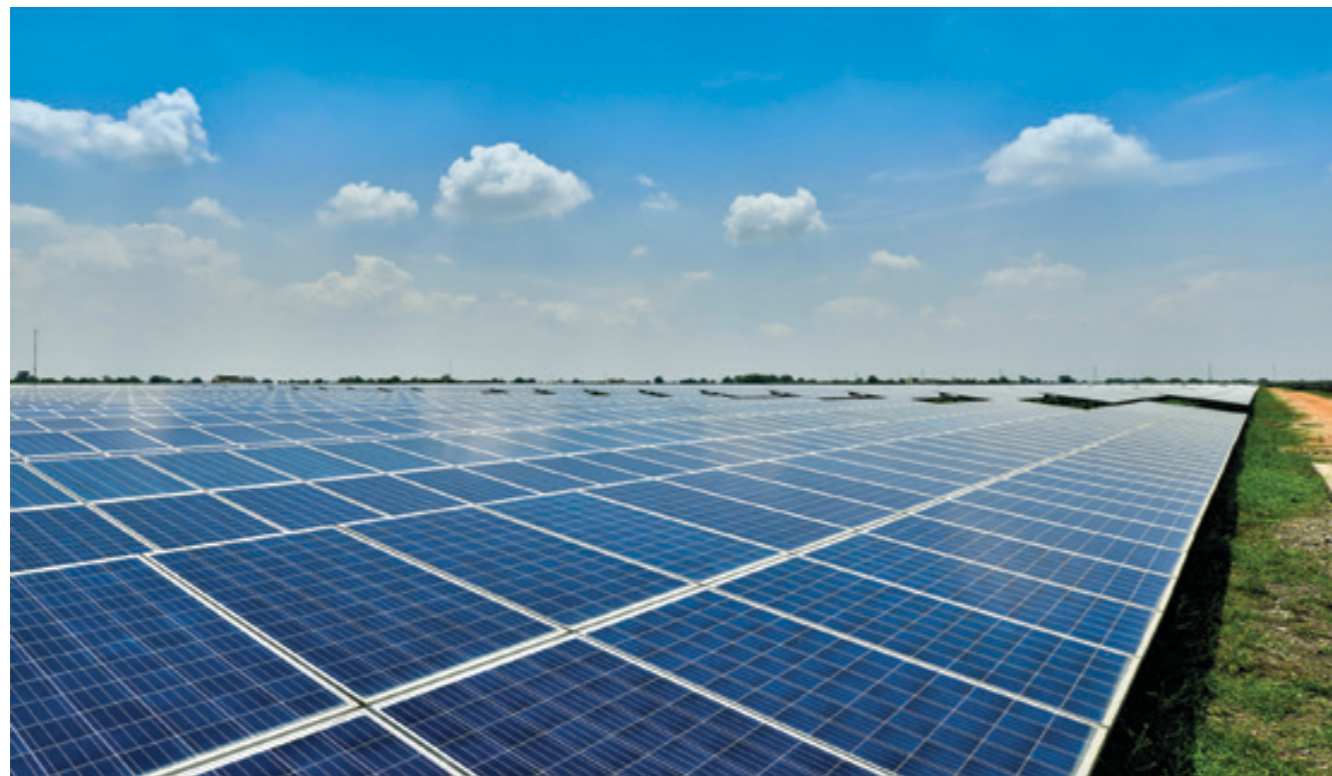
A 50 MW solar power plant installed by Sterling and Wilson Renewable Energy Limited for Giriraj Enterprises in Virudhunagar, Tamil Nadu
